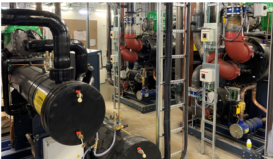
Ringsted installation of Geoclima heat pumps utilizing Danfoss Turbocor oil-free compressors with Solstice ze (R-1234ze) refrigerant. Image courtesy of Danfoss.
